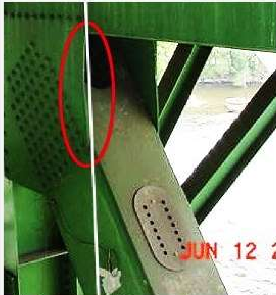
The ill-fated, warped U10 gusset plate on the I35W bridge. June 12, 2003.
